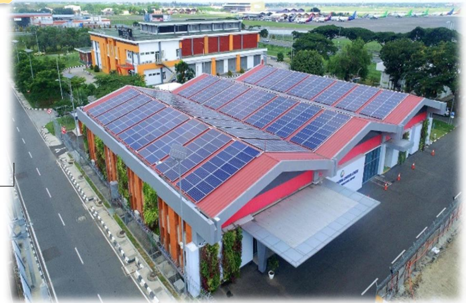
In AOCC (AirPort Control Operation Center) building Soekarno Hatta Airport COD October 2020
